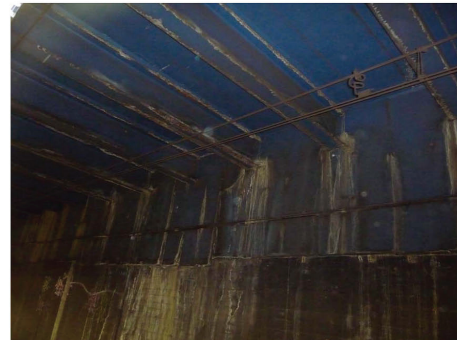
Image 3 - Deterioration of beams supporting ESR roof
